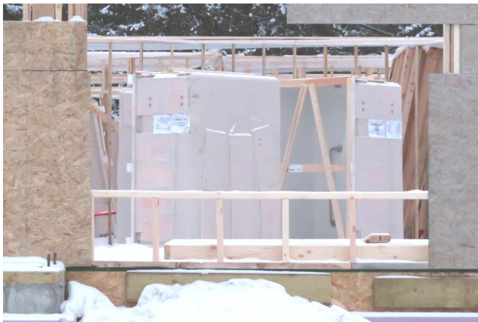
An note of interest: The shower units are already in the rooms!!
