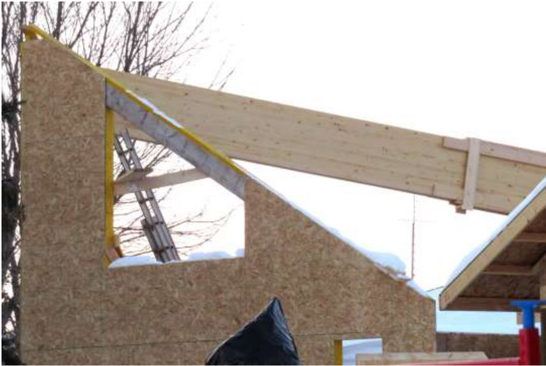
Huge beam put into place in the chapel, view from the front looking toward the northwest
